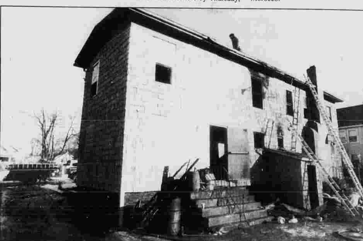
CAFE FIRE — Fire officials survey roof damage caused by a fire today at the Hartford Road Cafe, 378 Hartford Road. The fire has been termed suspicious.
